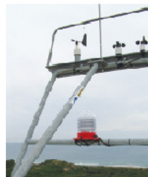
AV125 obstruction lights mark wind turbines in Gippsland, Australia
